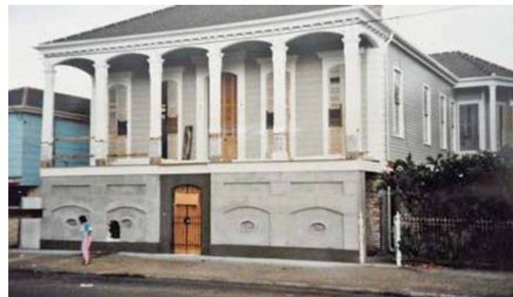
TOP: Early-1980s view of steel used to support a house during elevation project on Rampart Street.
